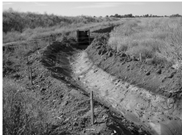
recently installed sediment trap in Yolo County
